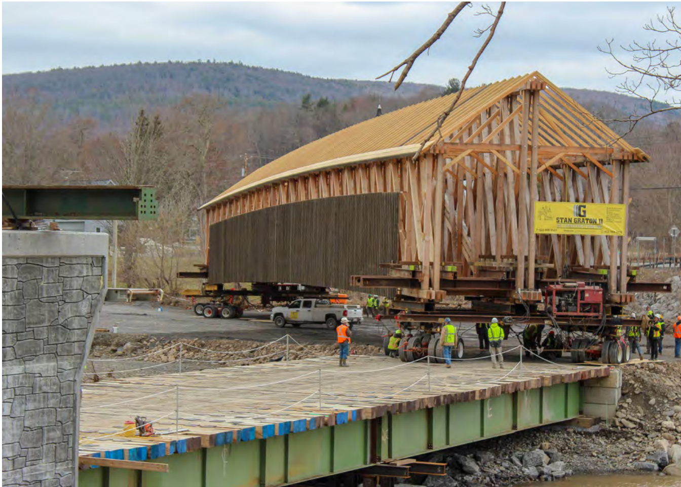
New covered bridge, turning the tight corner on to the onto temporary bridge
