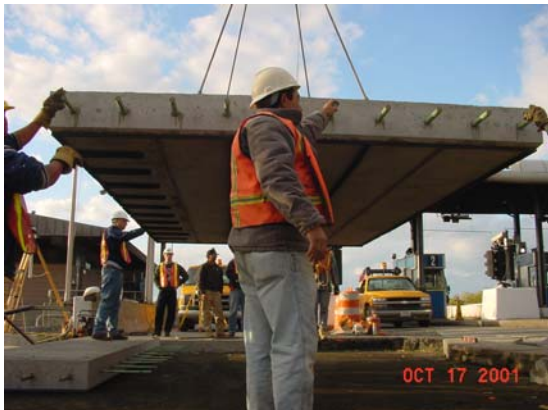
Figure 1 - 'Super-slab' precast pavement slabs at Tappan Zee Bridge Toll Plaza consisting of an interconnecting series of precast slabs that can be installed and placed into service immediately.
