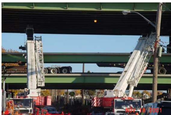
Figure 2 - Installation of 'Inverset Bridge System', Long Island Expressway /58th Street in Queens.
